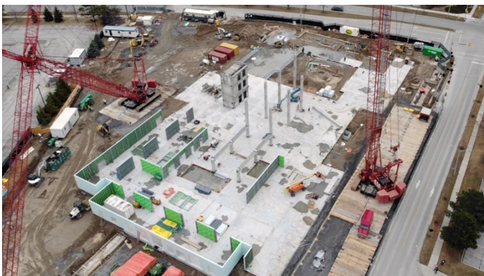
The first-floor walls and the elevator core taking shape just 24 days after the first photo was taken
