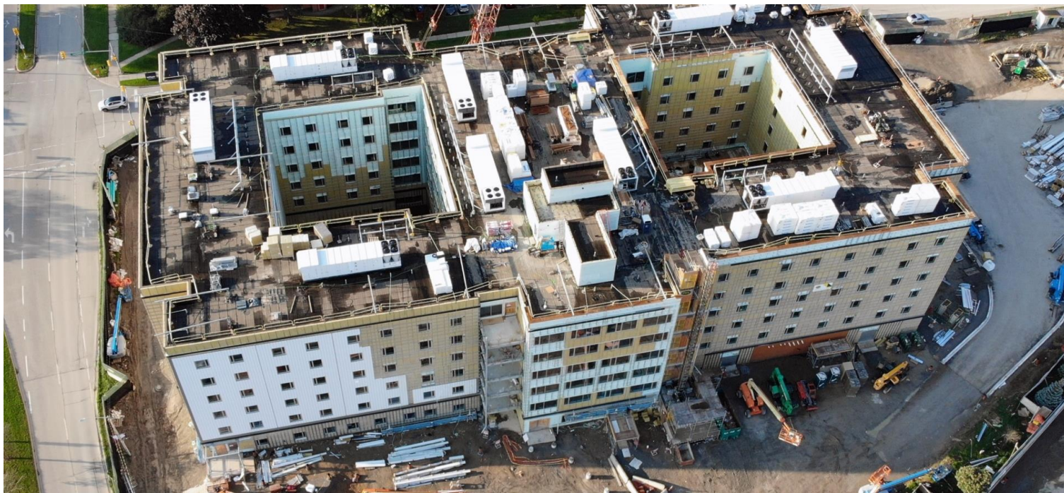
A look at the new exterior siding on the north side of the building (October 11, 2021)
