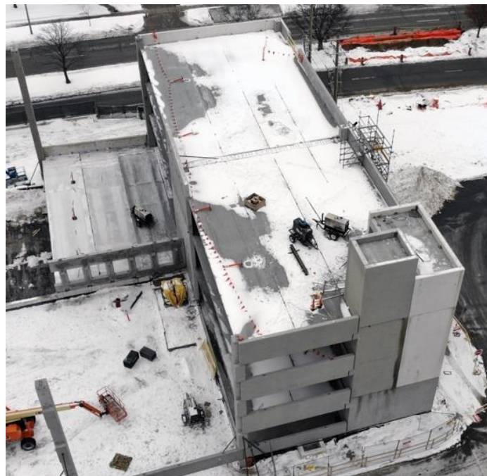
An aerial photo of the 500-spot parking garage in progress on February 6, 2022
