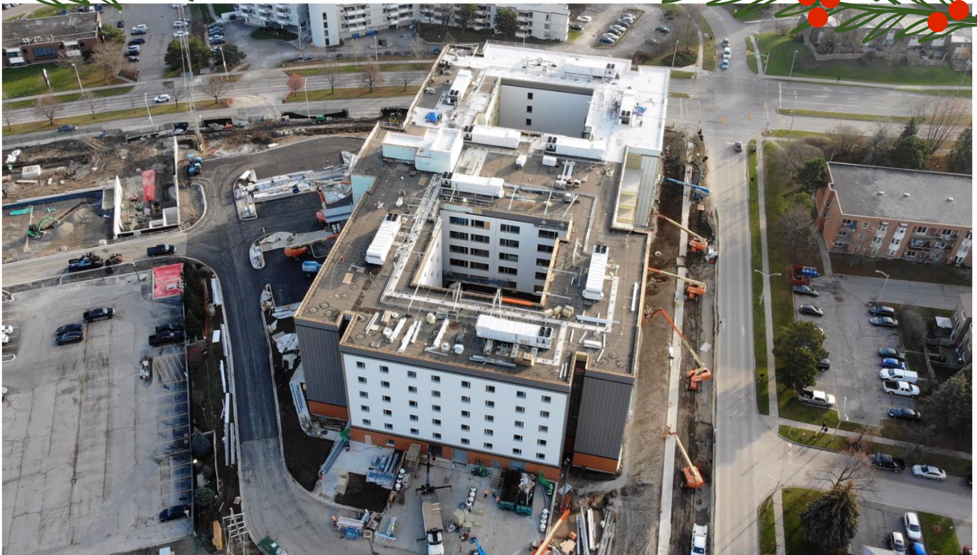
An aerial view of the home from the east side of the building on December 4, 2021. On the south side of the building, crews are finalizing exterior panel installation and the paved road network is complete on the north side. On the top left, the site of the future parking garage can be seen.
