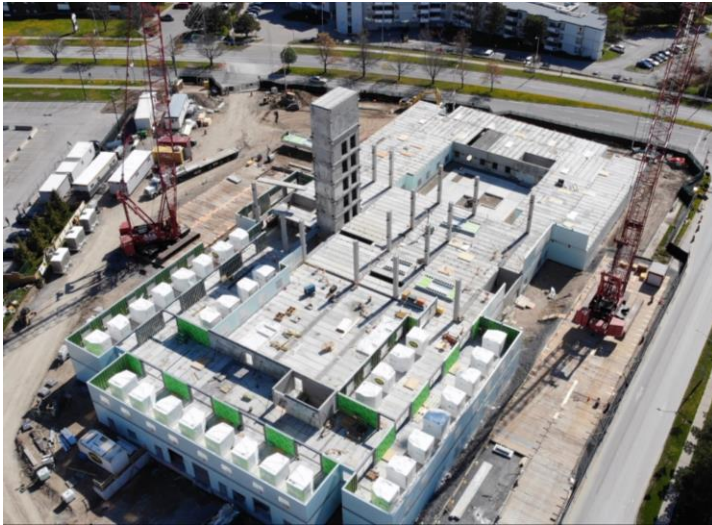
The completed elevator core and partially completed second floor with 32 washroom pods on May 8, 2021
